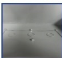
3 Knock Out Holes
